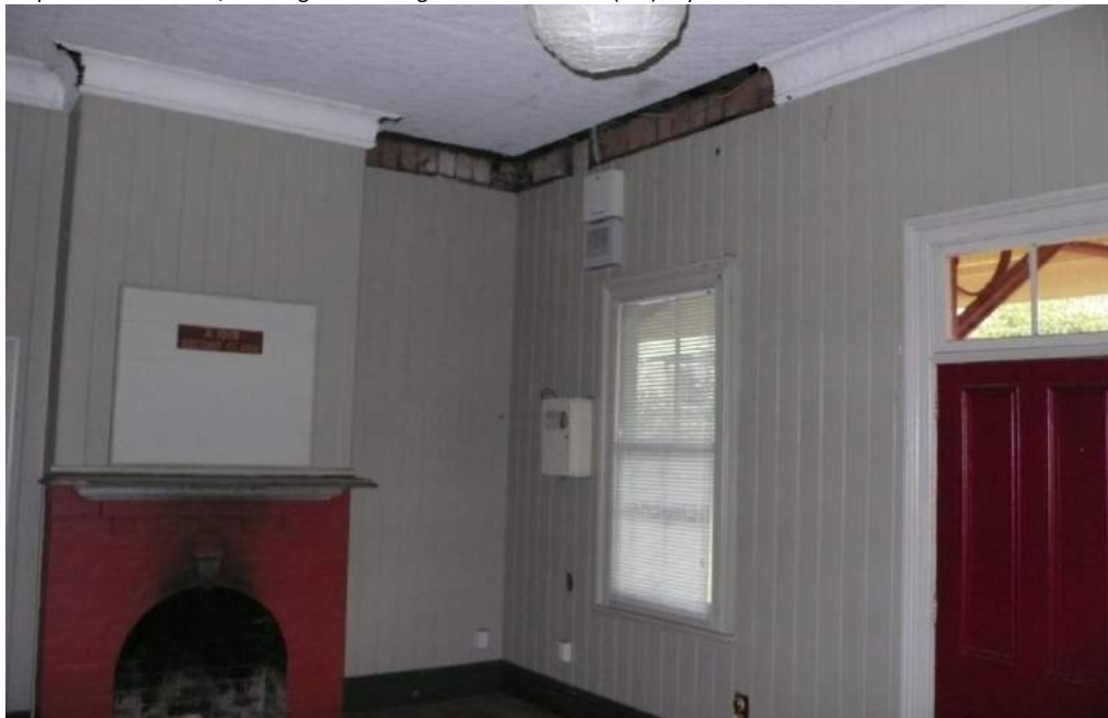
South west corner of the Station master & Booking Office, note large section of cornice missing, Images: B, T & K Architects 2015
