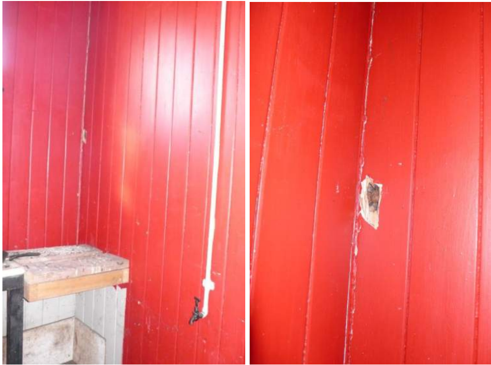
Showing north east corner of kitchen area + wall mounted tap (left) damage to t & g wall lining
