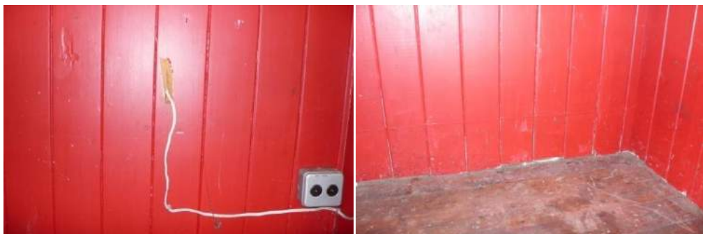
Exposed wiring (left) missing skirting board in kitchen
